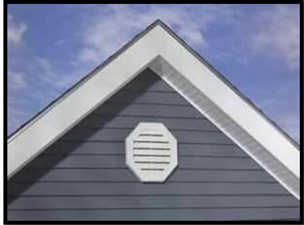
Figure 16 – Example of a faux gable vent for decorative purposes only.
