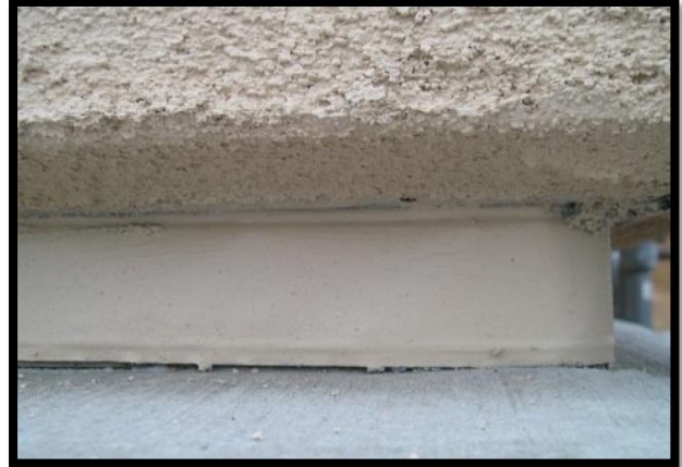
Figure 24 – Example of the base of the siding properly sealed with stucco and flashing to prevent exposure to the base of the house.
