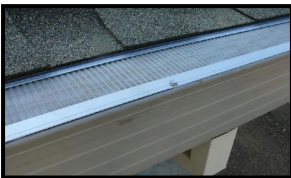
Figure 17 – One example of a gutter cover or guard to protect against debris accumulation.
