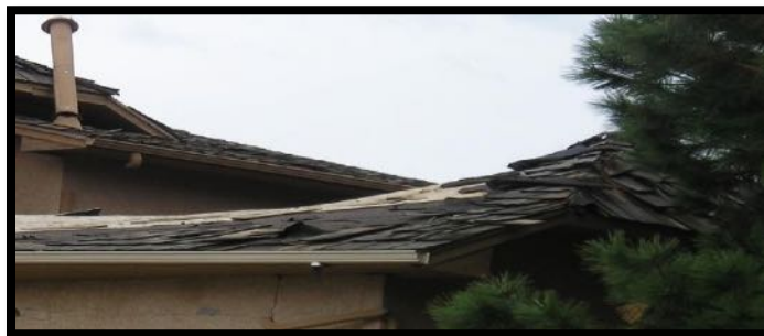
Figure 1 – Example of a shake shingle roof that was ignited from an ember in the 2012 Waldo Canyon fire.
