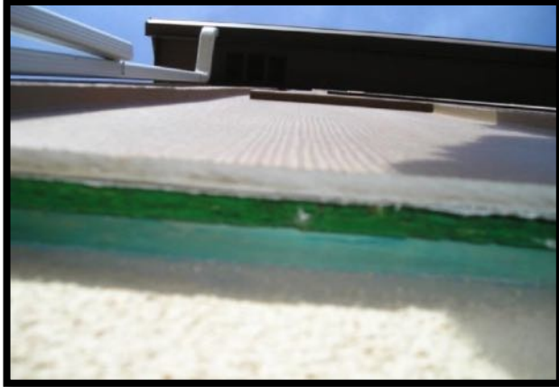
Figure 23 – Example of the base of a wall that reveals exposed plywood and insulation where the foundation and siding meet at the base of the house.
