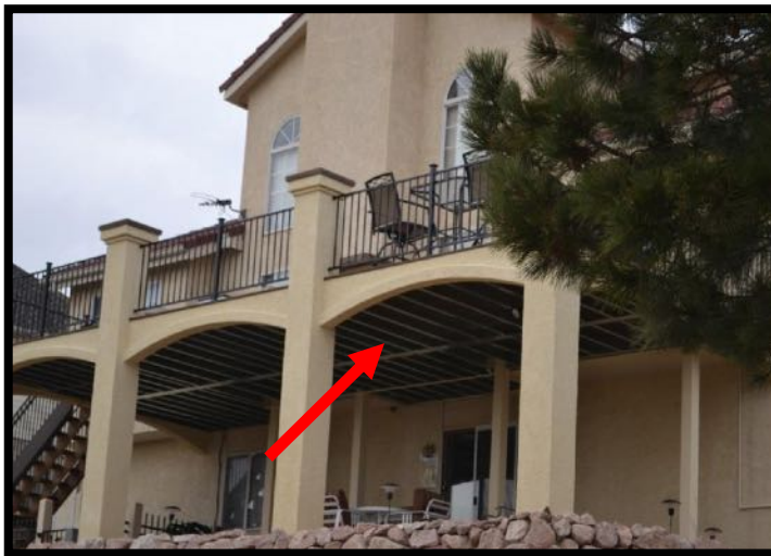
Figure 22 – The arrow depicts the metal floor joists used on this example deck.
